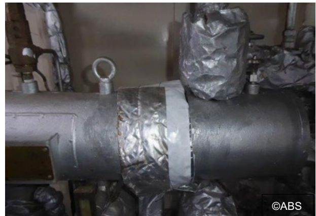
Fuel oil purifier flange isolated with band
