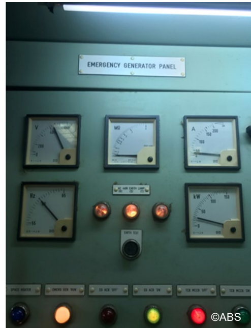
Emergency power auto start not functioning
