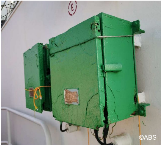
Electrical control boxes found broken
