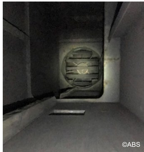
Engine room fire damper found defective
