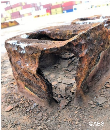
Wasted container socket - before
