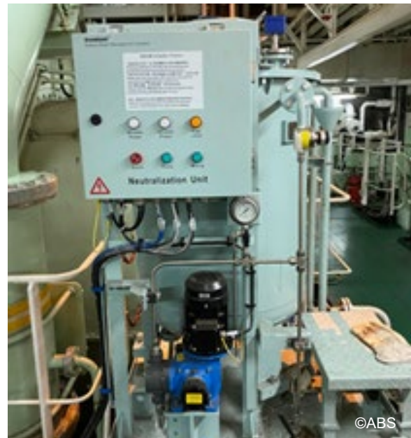
Ballast Water Treatment System found inoperable
