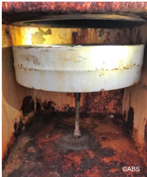
Air pipe float found defective
