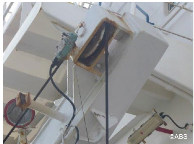
Lifeboat limit switch malfunction
