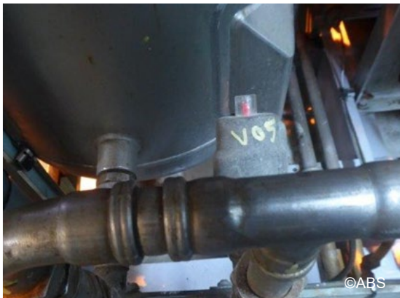
Oily water 3-way valve not functioning
