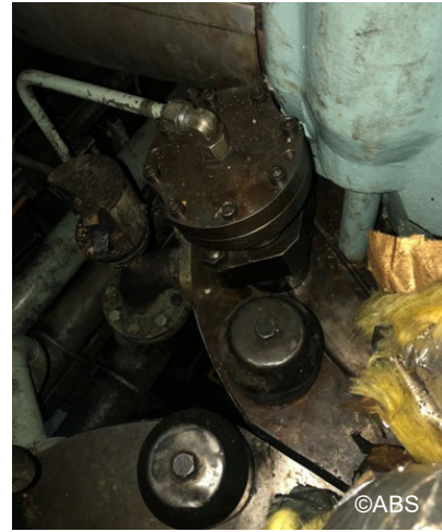
Faulty Starting Valve replaced by spare
